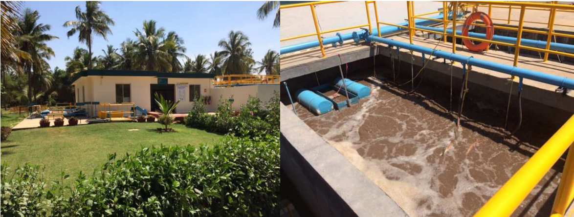
Overview of Combined Treatment system ↑
