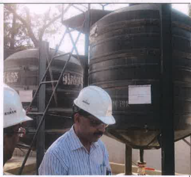
View of tanks to store the effluents
