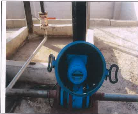
View on Flow Meter
