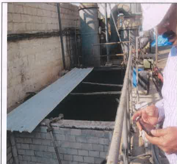
View of tank below GL to store effluents
